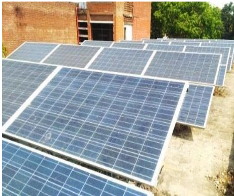
Solar panels in the college
